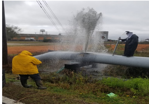
Chris Smith and Gage Allen of the Maintenance department repairing the force main at the PMP plant located on the river road bridge crossing.
