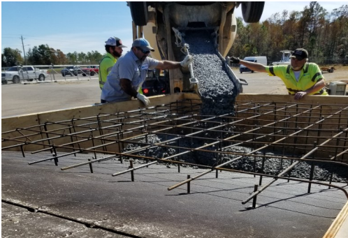
Walker Riley, Mike Newbill, & Wilberto Luciano of the Maintenance department pouring new slab for the generator and fuel tanks at Hwy. 63 location.
